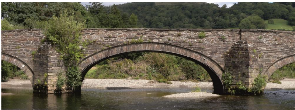
FIGURE 2 THE CENTRE SPAN WITH AN ELLIPTICAL CURVE OVERLAYED. NOTE THE SHOULDERS SITTING CLEARLY ABOVE THE LINE INDICATING A 3 CENTRED CURVE
